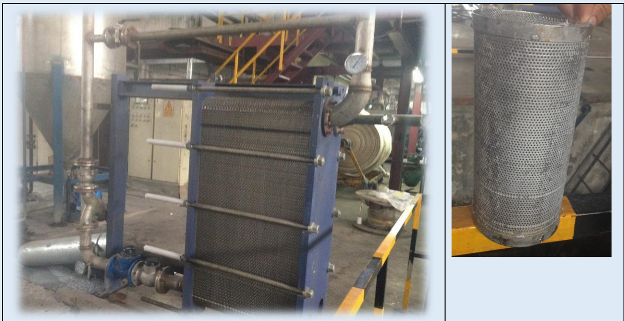
Figure-22: Plate heat exchanger for heat recovery from composite textile wastewater
