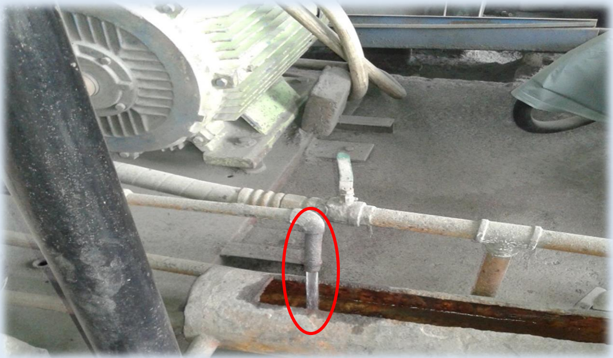
Figure- 14: Cooling water discharge from the therm oil heater pump
