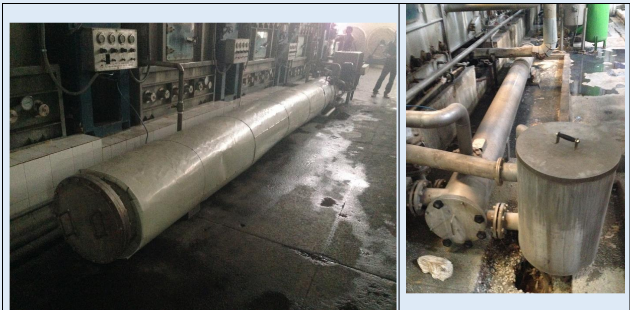
Figure- 21: Shell and tube heat exchanger directly installed at continuous pre-treatment machines (two different machines)
