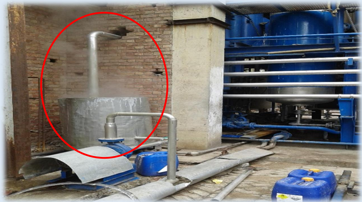
Figure-6: Vapor condensate from CRP is collected at over ground tank and then supplied to the pretreatment machine for post bleaching washing
