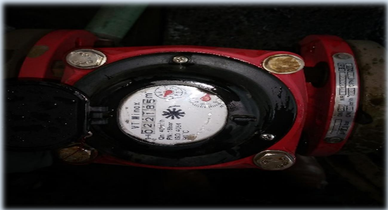
Figure- 18: Water flow meter installed at boiler feed water supply line
