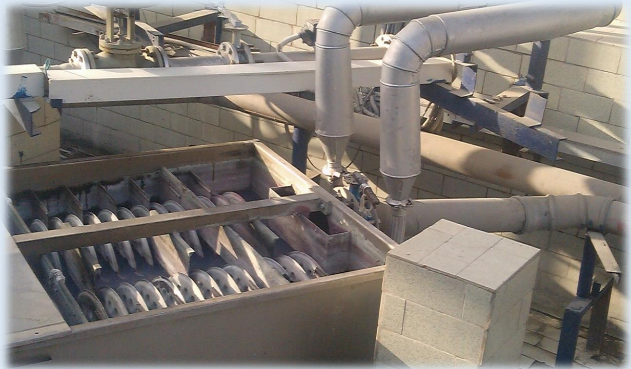
Figure-23: Disc heat exchanger for heat recovery from composite textile wastewater
