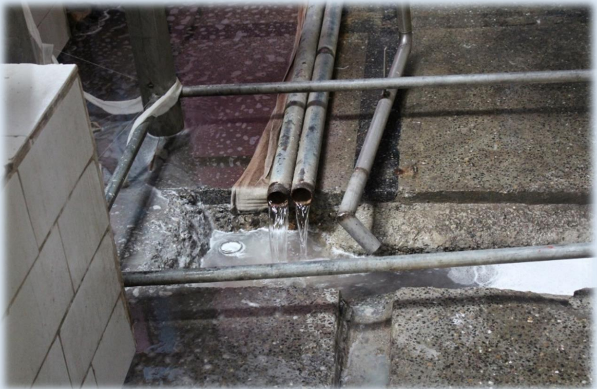
Figure-2: Cooling water wastage from singeing machine
