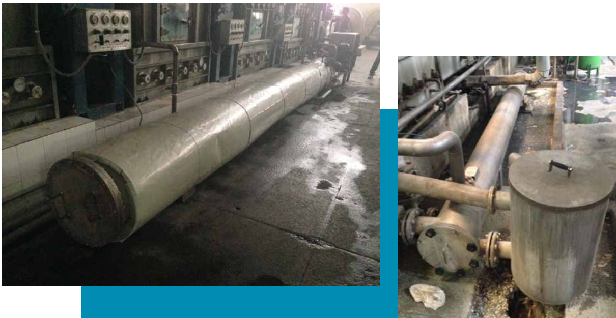
Figure-21: Shell and tube heat exchanger directly installed at continuous pre-treatment machines (two different machines)
