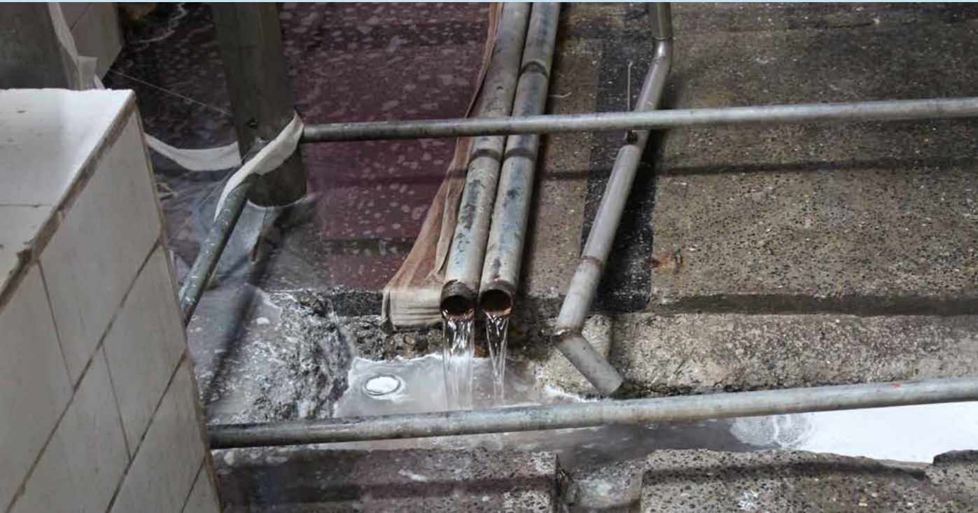
Figure-2: Cooling water wastage from singeing machine
