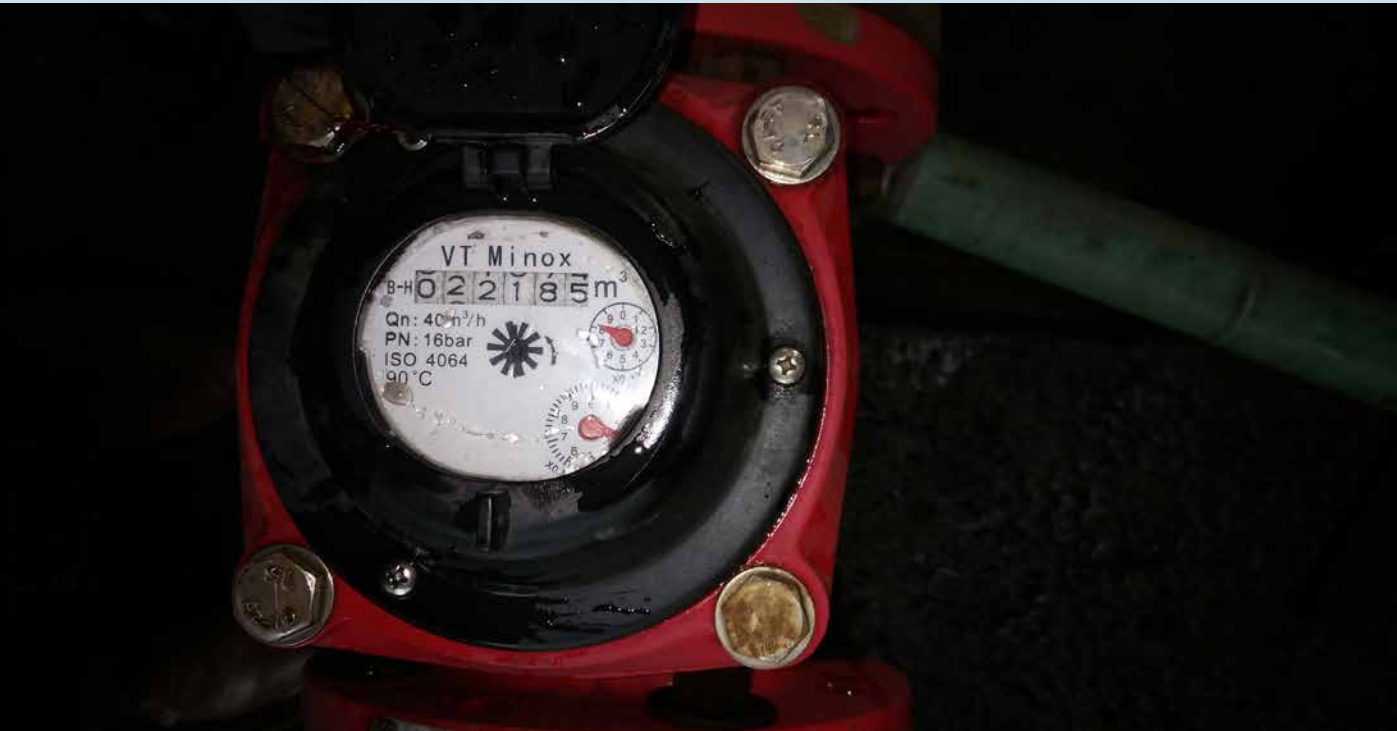
Figure-18: Water flow meter installed at boiler feed water supply line
