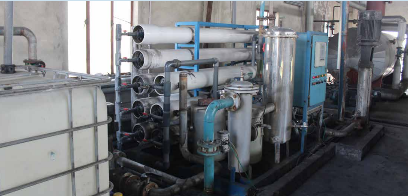
Figure-1: Reverse osmosis plant for preparing water for wet finishing processes and boilers
