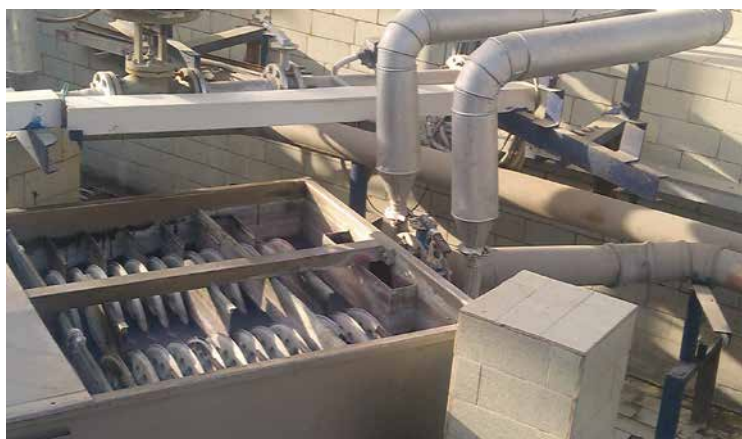
Figure-23: Disc heat exchanger for heat recovery from composite textile wastewater
