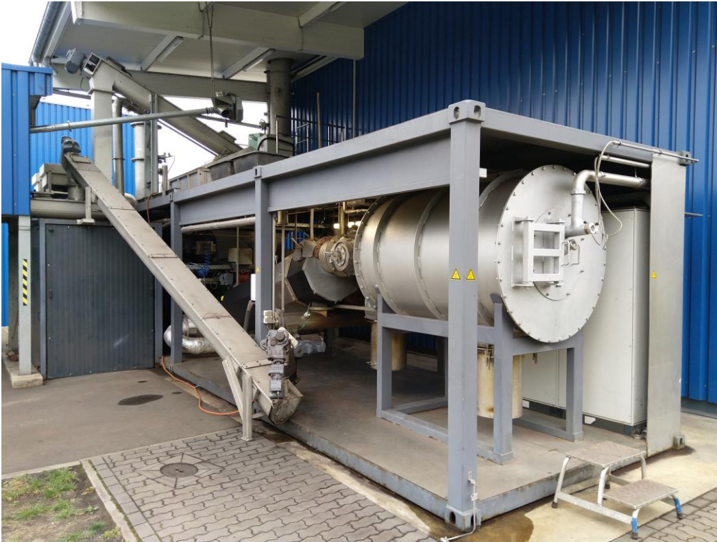
Figure 8: Sludge Pyrolysis Unit for Char Production
