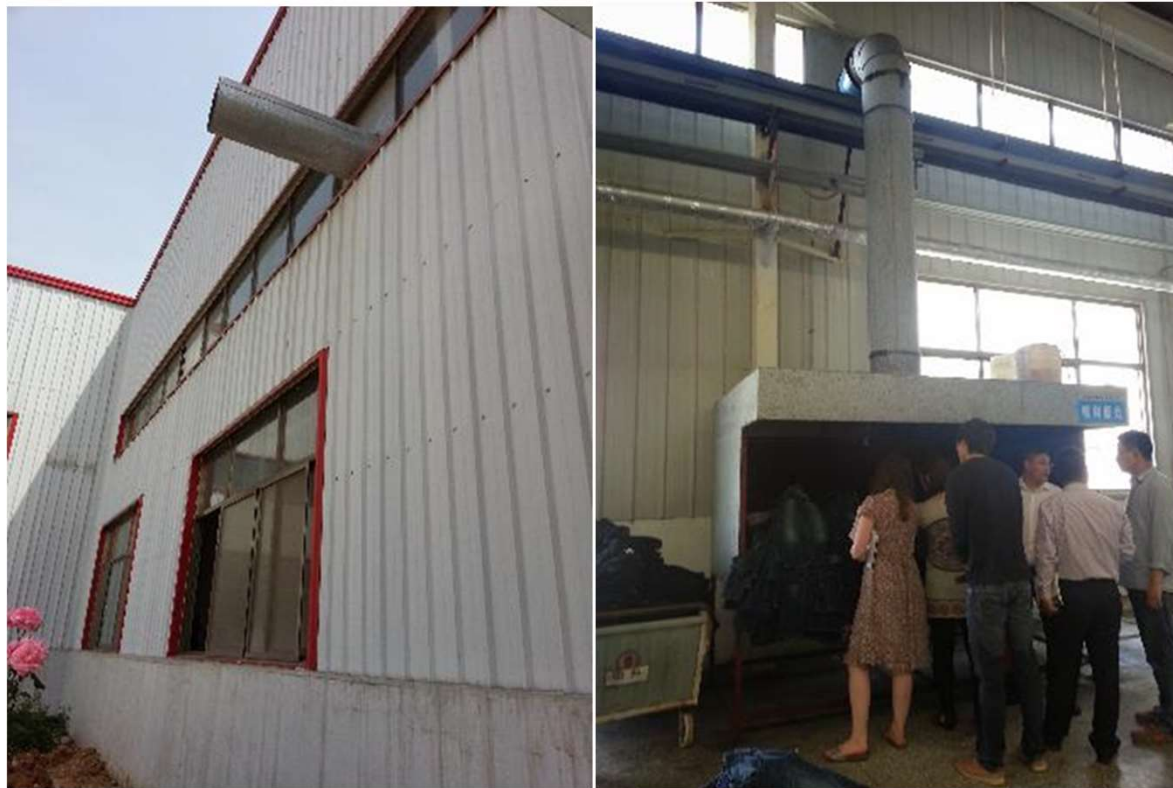
Fume hood for resin spraying in a denim laundry
